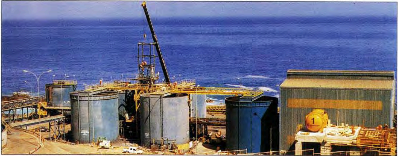
Slurry receiving tanks at Coloso.
